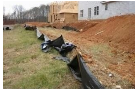
Silt Fence Fail
