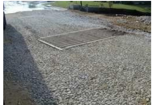
Stone Construction Entrance with Washrack
