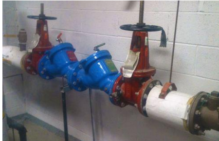
Figure 9 – Example of a Backflow Prevention Assembly
